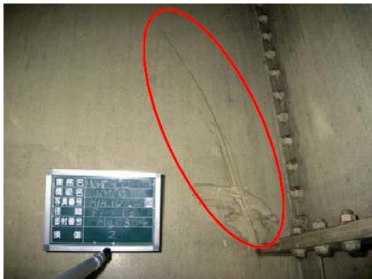
Fig. 2 Crack on Yamazoe Blidge
